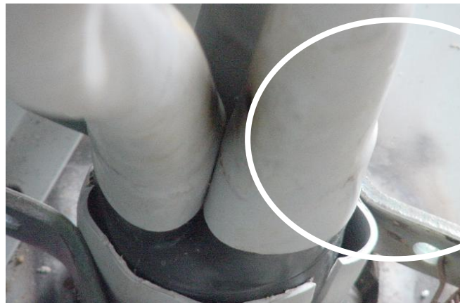
Figure 2. Example of signature of insulation failure due to electrical tree
