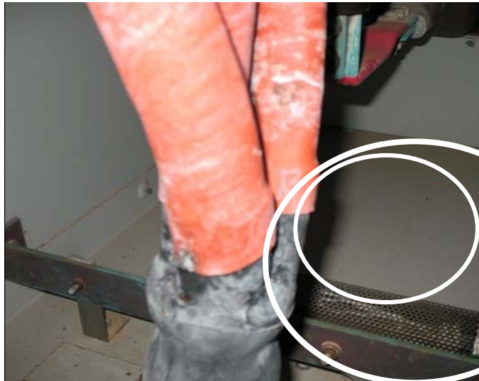
Figure 1. Example of surface tracking at a cable termination
